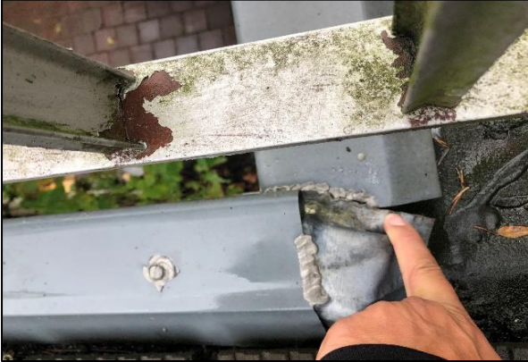
7. Openstaande verbinding tpv dakrand.
