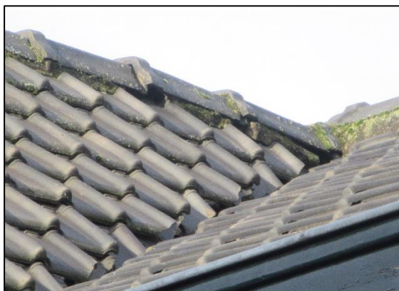
4. Poreuze cementlaag tpv nokvorsten.
